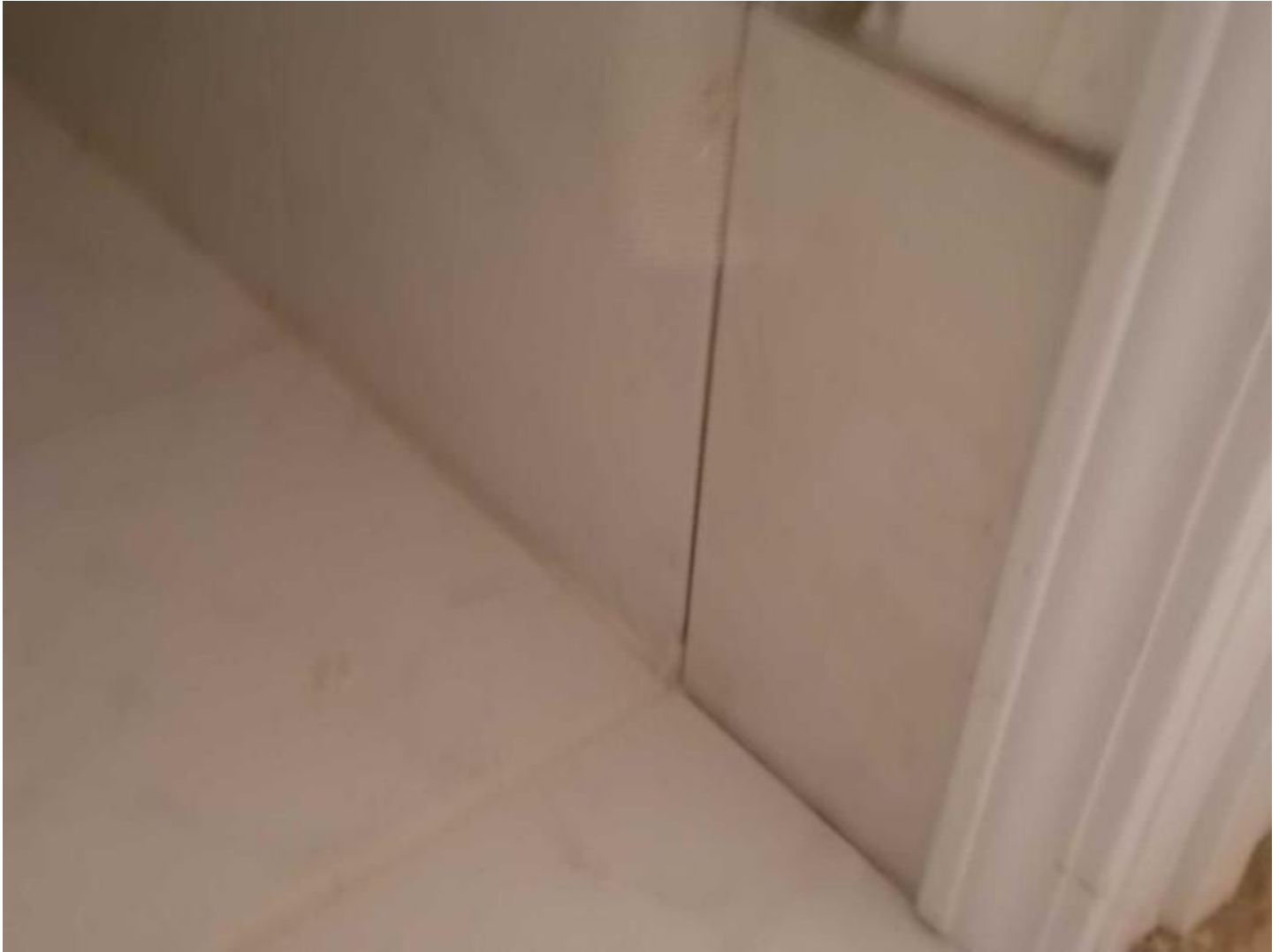
18 DSCN0035 Date Taken: 3/12/2015 Taken By: George Niezgoda Utility closet ceramic base that was not sealed
