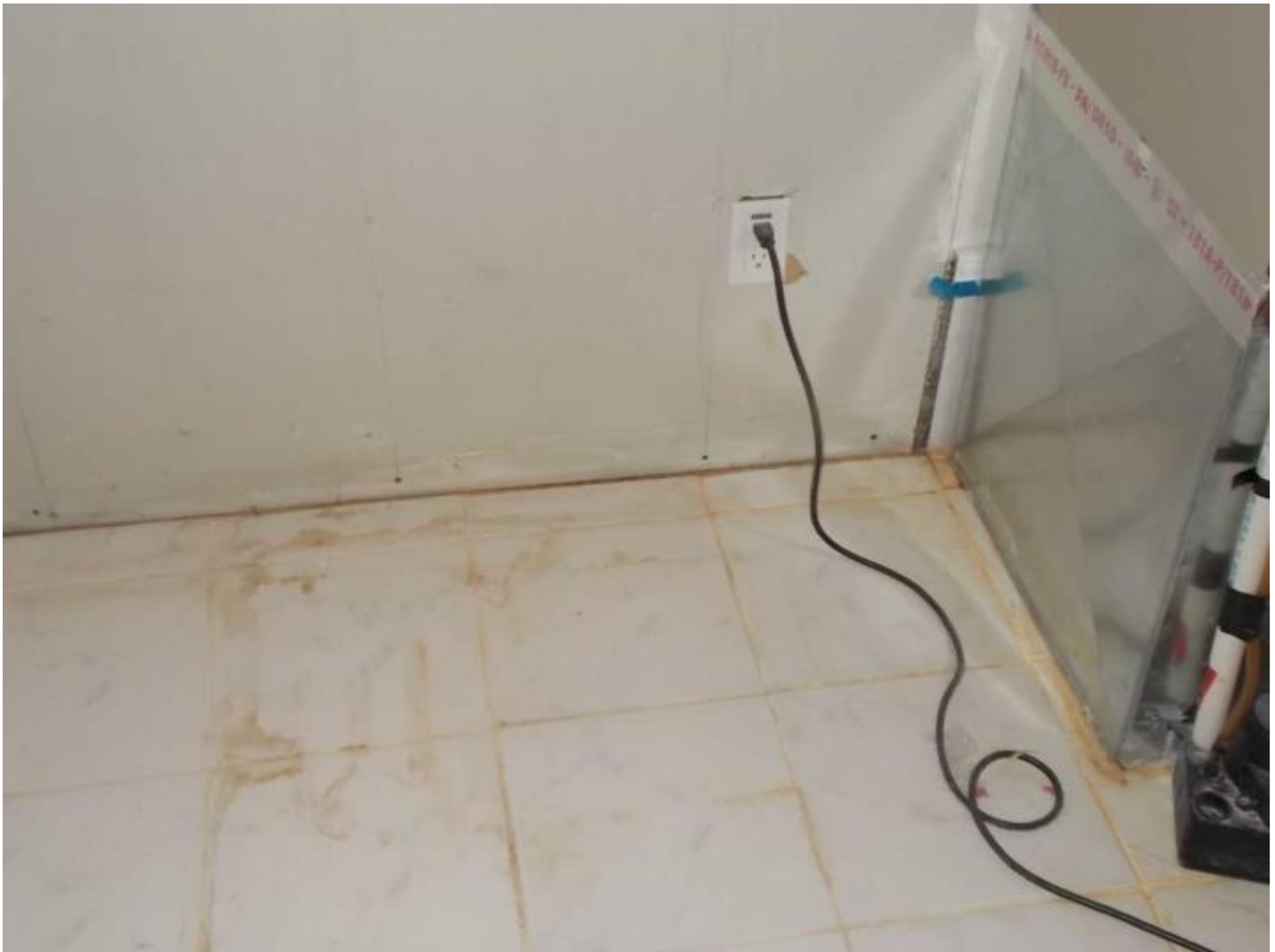
8 DSCN0029 Date Taken: 3/12/2015 Taken By: George Niezgoda Water staining on drywall in utility closet
