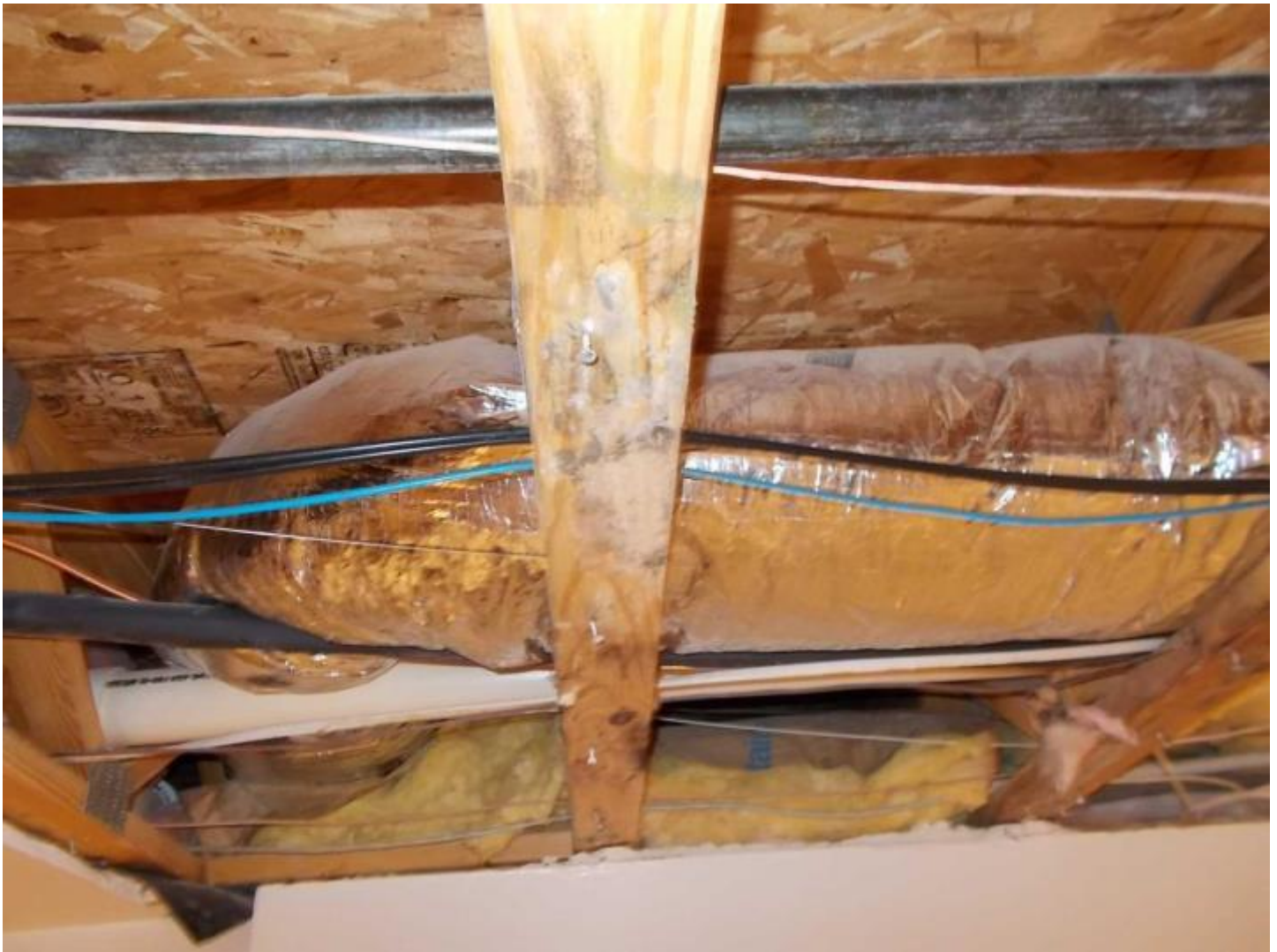
1 DSCN0020 Date Taken: 3/12/2015 Taken By: George Niezgoda Visible mold like growth on the rafters in the kitchen.
