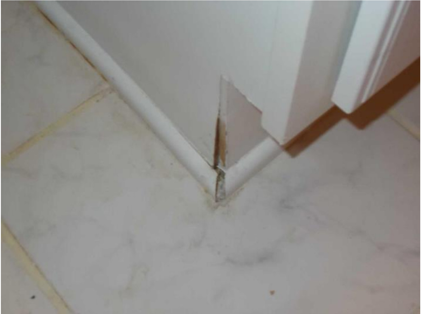
17 DSCN0036 Bathroom Vanity swollen at bottom
