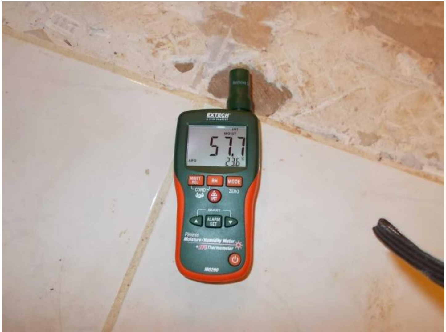
4 DSCN0025 Date Taken: 3/12/2015 Taken By: George Niezgoda Tile floor in kitchen elevated moisture
