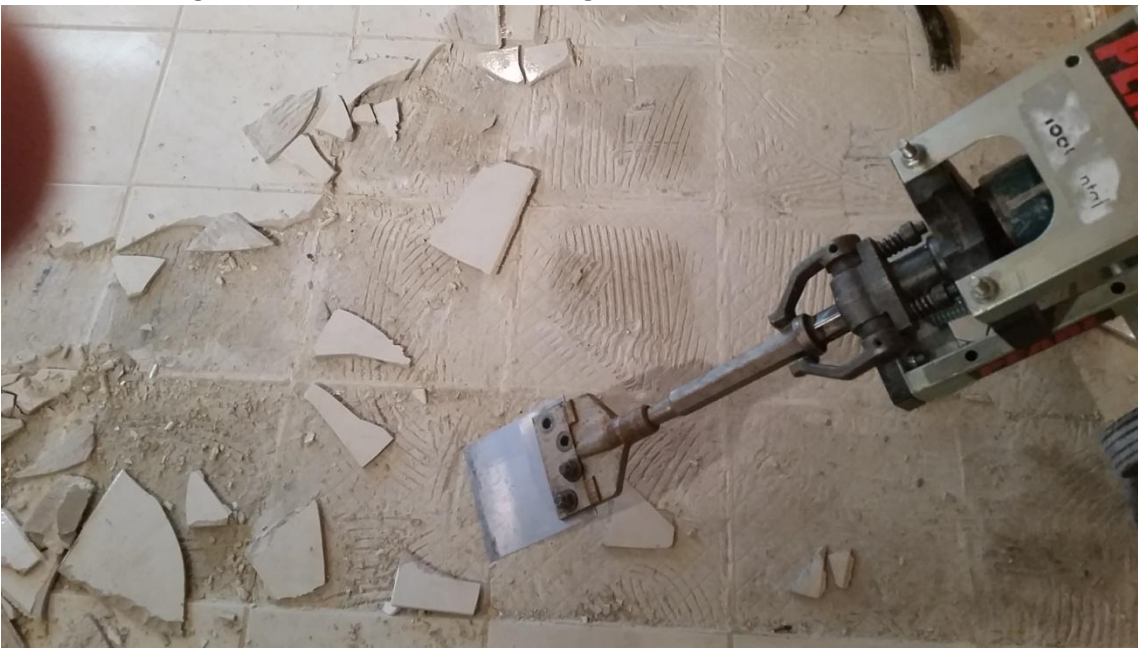
On or about 4/28/2015; Evidence that moisture was still under tile floor (resulted in high moisture readings) Evidence that moisture still existed under the tile floor and was not properly dried by Servpro resulting in high moisture readings which was the cause of mold growth
